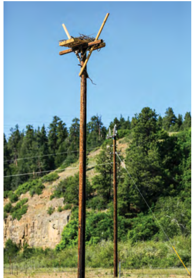
Raptors were building a nest on the energized pole in the background, but have now been relocated to their own “bird condo.”
