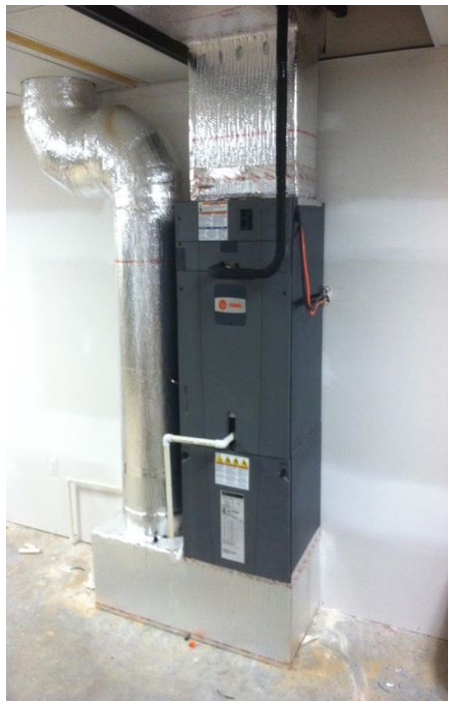
Central Air Handler
