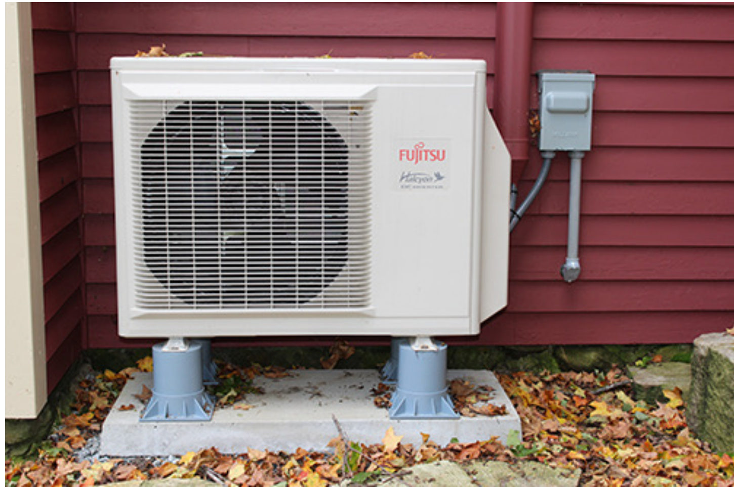
Air Source Heat Pump
