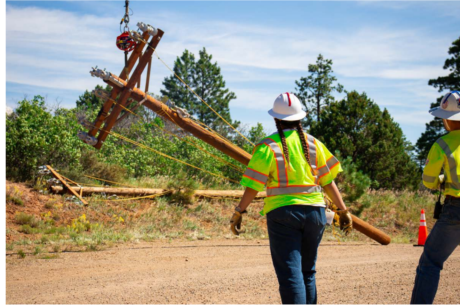
LPEA Intern Katie Killinen and staff John Keating assist with the helicopter pole placement.
