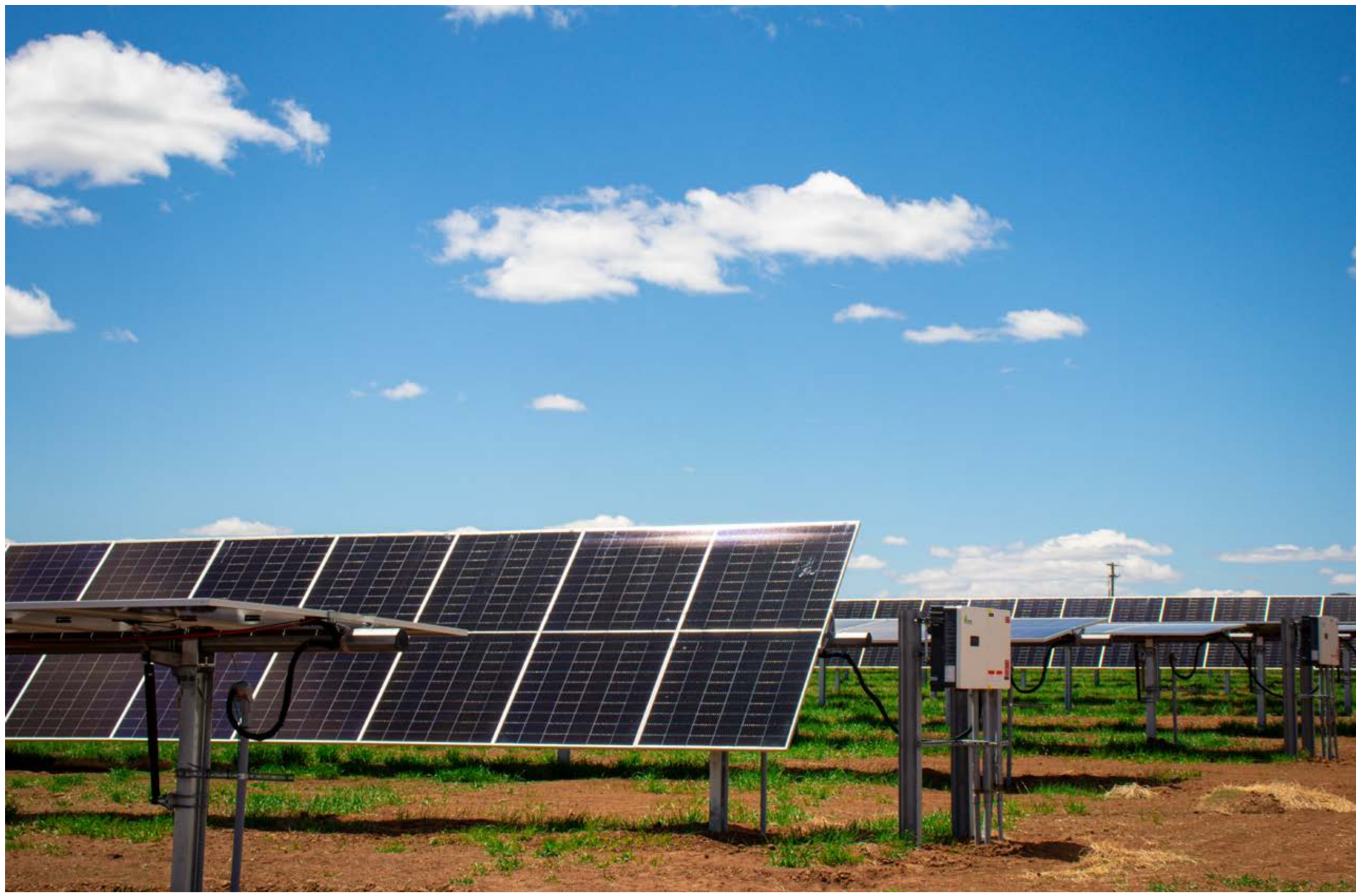
The Sunnyside Solar array construction began, including 3,627 panels situated on 9 acres off Highway 550 near Sunnyside Elementary in Durango. This constituted the first cooperative-owned community solar project.
